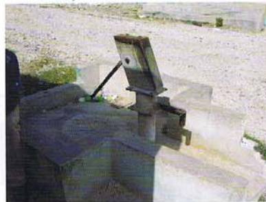
An existing water well in one of the communities included in the project, with hand pump, now completely dry, closed and out of use
